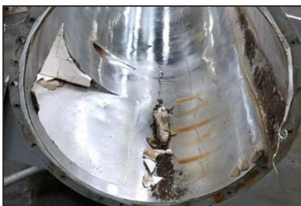
Signs of abrasive wear to internals of mixer.
