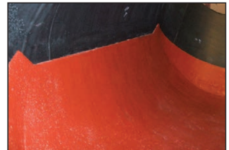
Repaired unit ready for install.
