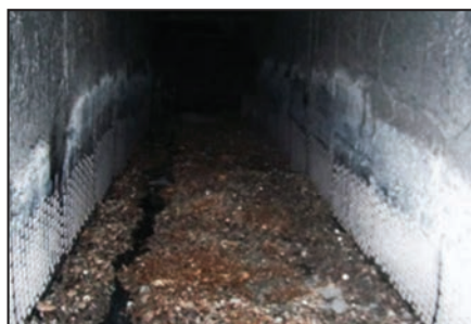
Discharge flume with damaged tile/rubber liners.
