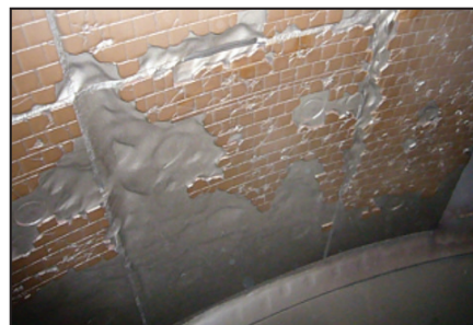
Damaged pulverizer walls.
