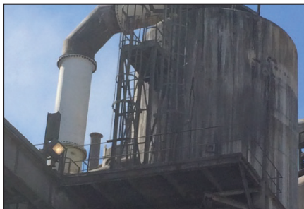
Flash cooler with exhausters.
