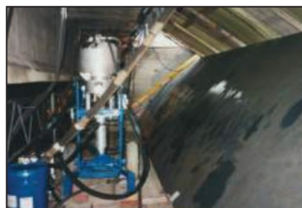
Pitting repaired using ARC 858 .
