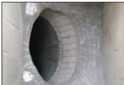
Damage to existing ceramic tiles caused unscheduled shutdown and loss of production.
