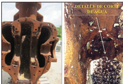
Pump body as inspected.
