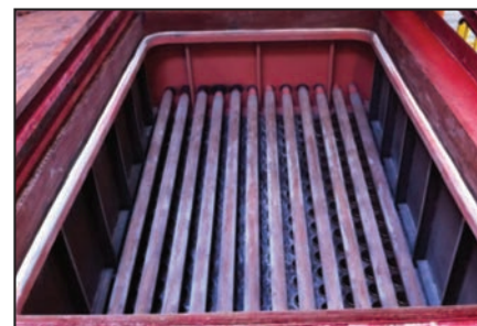
Bag house protected with ARC S7 in service over 2 years with no failures.
