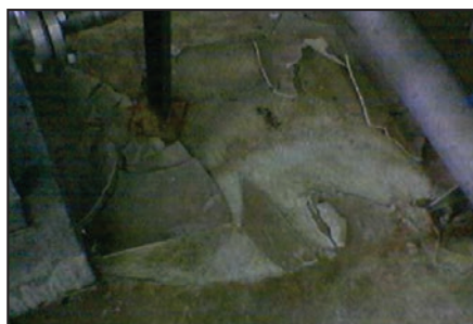
Delaminated fiberglass mat polyester.
