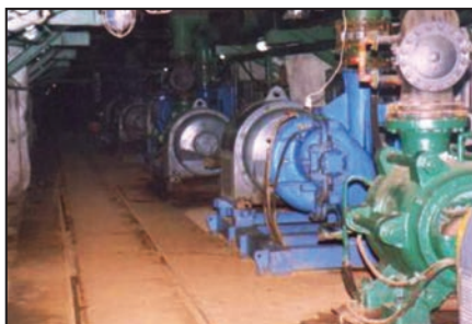
Bank of dewatering pumps.
