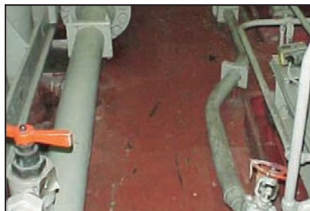
Previous coating one year after installed.
