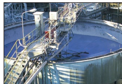
ARC S2 still in excellent condition.
