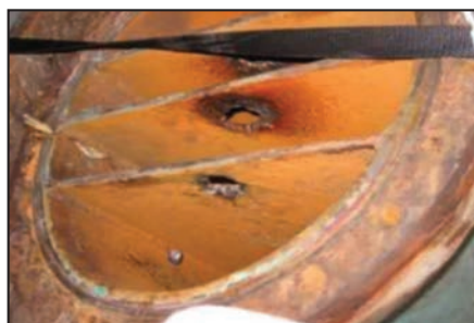
Corroded divider plates.
