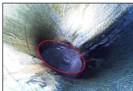
Dark scale formation on unlined section.
