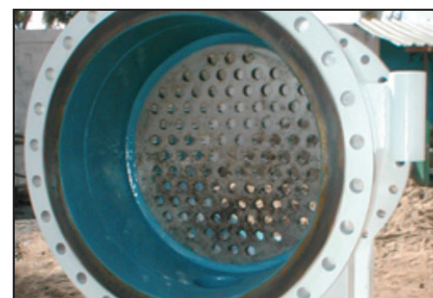
After cleaning and decontamination, ARC 858 is applied to fill and smooth surface.
