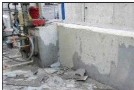
Failed coating after spills.
