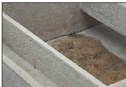
Drained sand filter vessel.
