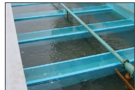
Sand filter in service.
