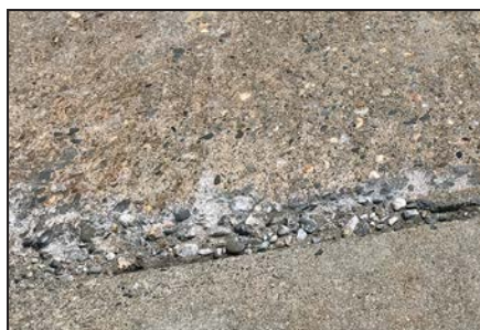
Damaged concrete surface.
