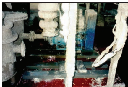
ARC 988 coated pump base: good condition after four years.
